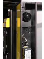
Security alarm system
